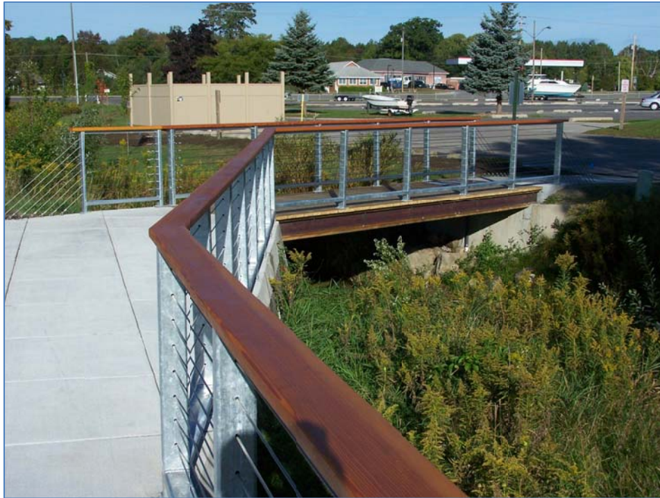
Photo: Gosling Czubak Engineering Sciences, Inc
