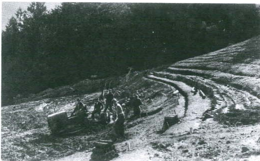
FIGURE 35. In April 1934, construction began. With the only earthmoving equipment ever used on the site, enrollees re-graded the stage, installed drainage and water supply lines and began the rough terracing of the lower seats, following the alignment of the existing 1929 row (MV/PL).
