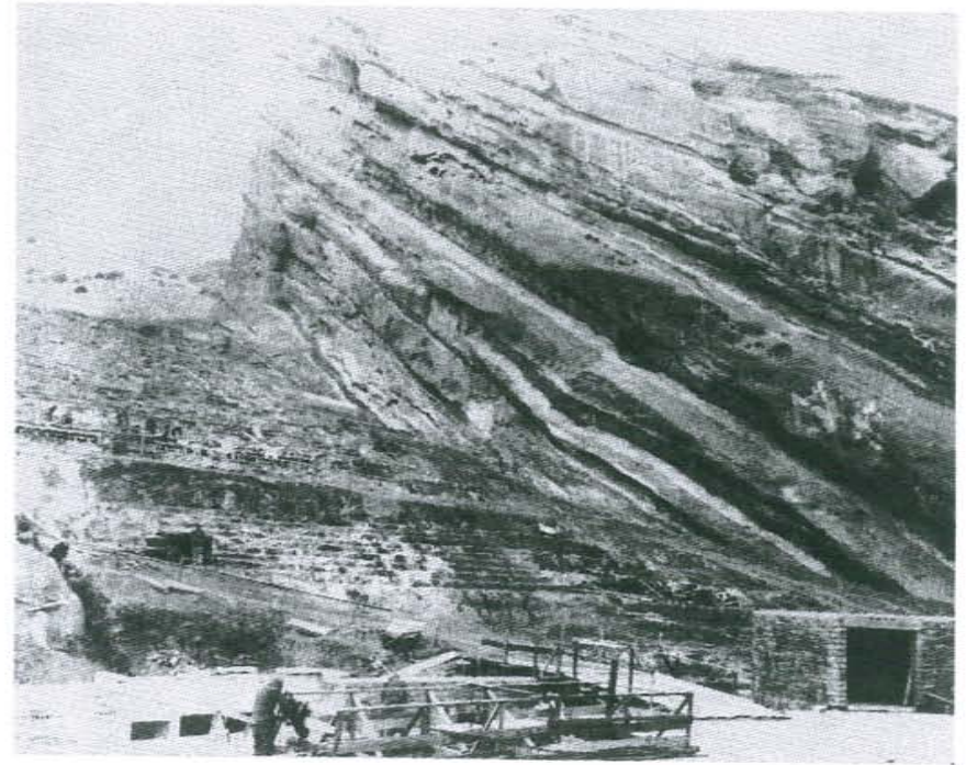
FIGURE 21. Mid-1937. To create the auditorium, enrollees cut as much as 28 feet from the upper north side, revealing a protruding ledge. Rather than try to blast away the ledge, Hoyt and Morse realigned the theatre breaking with the original symmetrical plan (BBMM).
