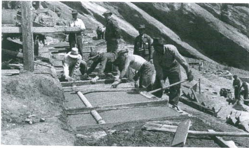
FIGURE 20. 1938. Like the planters, the seating was designed by sketching, building an in-place prototype, and then adjusting and drawing the detail. Here enrollees form the gutters that carry storm water along the 3.33% slope across each row of seats (DPL).
